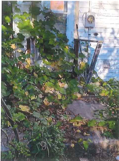
A secondary entrance to the house at the rear of the property has a dilapidated deck in front of the door. The structure is unsafe and needs to be removed and replaced.
