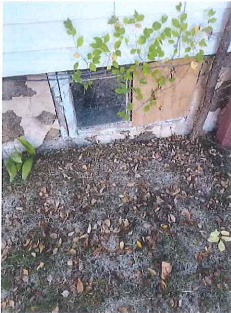
Broken basement window has plywood covering the opening. Window needs to be removed and replaced.
